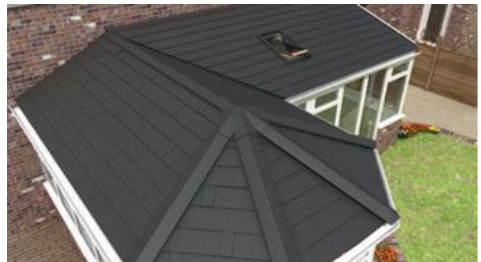
Chosen tile is added ensuring weathertightness and the gutter and external trim are secured in place.
